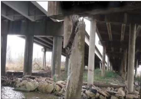
THIS CONCRETE PIER, under the westbound lanes of I-10, was struck by an uncontrolled barge. TxDOT reported a structural failure both above and below the water line. They reported that they will let an emergency contract in a few days, for repairs and/or replacement of the pier. (Photo by We All Nosey)
