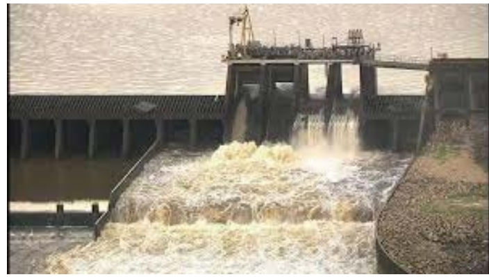
The existing flood gates consist of two radial gates used to release high volumes of water and two flashboard gates to accurately affect water levels on Lake Houston.
