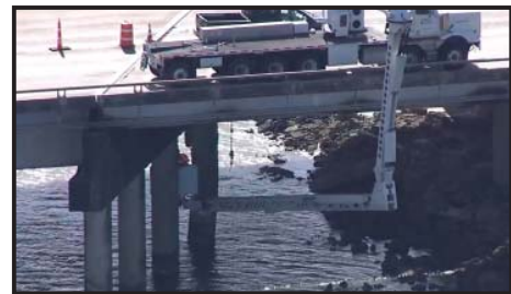
TxDOT workers examine the broken support.
