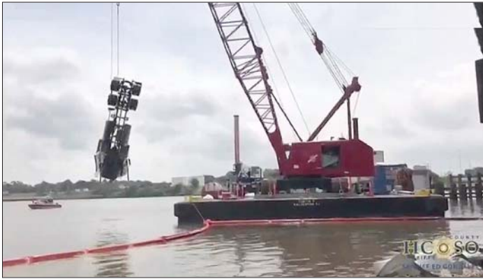
THE FRAME AND CAB OF THE SEMI truck that plunged into the San Jacinto River last Thursday, June 26 are lifted by a crane on a work barge on Saturday morning. The barge came from T&T Salvage in Galveston, and was required because the bridge and the nearby Waste Pits Superfund site were not suitable for this type of heavy lifting.
