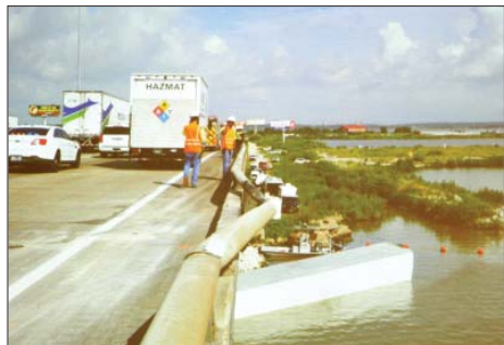
TxDOT workers inspect the damaged railing and view the 18-wheeler lying in the river, near the Waste Pits.
