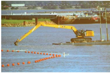
Contractors working for the PRP attempted to make repairs to the containment cap last month, but were working outside the Waste Pits site as defined by the red marker buoys.
