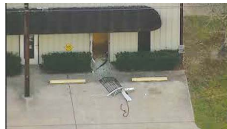
Burglars tore the door off the front of the building by chaining it to a pickup and pulling it out.
