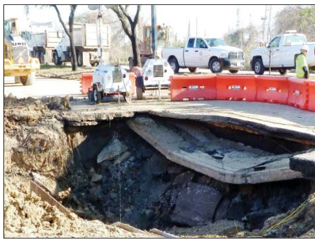
BROKEN PIPE IS UNDER REPAIR ALONG CLINTON DRIVE NEAR THE EAST LOOP.
