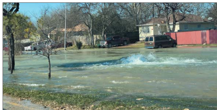
PICTURED TO THE LEFT: SITE OF THE BURST 96 INCH PIPE AT CLINTON DRIVE AND N. CAROLINA.
