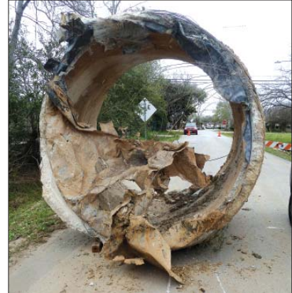
THIS IS THE SECTION OF OLD PIPE THAT FAILED AND FLOODED THE STREETS.
