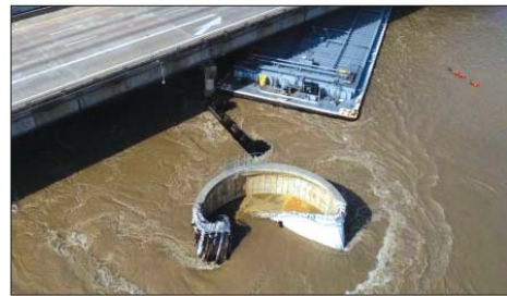
The Dolphin bumpers are badly damaged by the flooding and barge strikes, but are not due to be replaced for two years.
