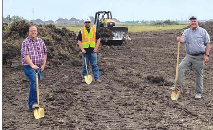
Front (L-R) County Engineer Cory Taylor and Commissioner Pct. 3 Gary Nelson on the back a Texas Sterling foreman at the groundbreaking of the new construction.
