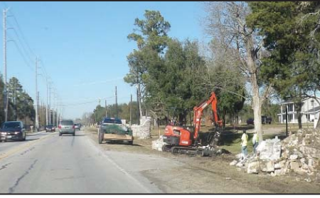
Centerpoint Energy put in new towering power lines at left along Main Street in Highlands. Next some gateway walls are being demolished to make way for a five lane highway to Barrett Station.
