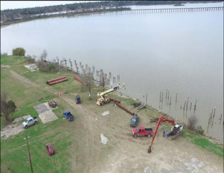
Construction activity along River Road includes piles about to be driven into the water to support a new set of berths for barges. To the left is Meadowbrook Park, and to the right the old Riverside Inn.
