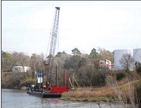
Piles are being driven across the river from the Waste Pits Superfund site, to repair and expand a fueling facility. Above the dock can be seen two storage takes, and buildings along Crosby-Lynchburg Road.
