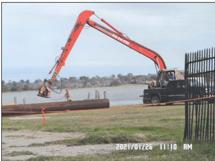
A pile driver and another crane are on site of the new Barge facility, ready to place and drive the steel piles shown under the crane arm.
