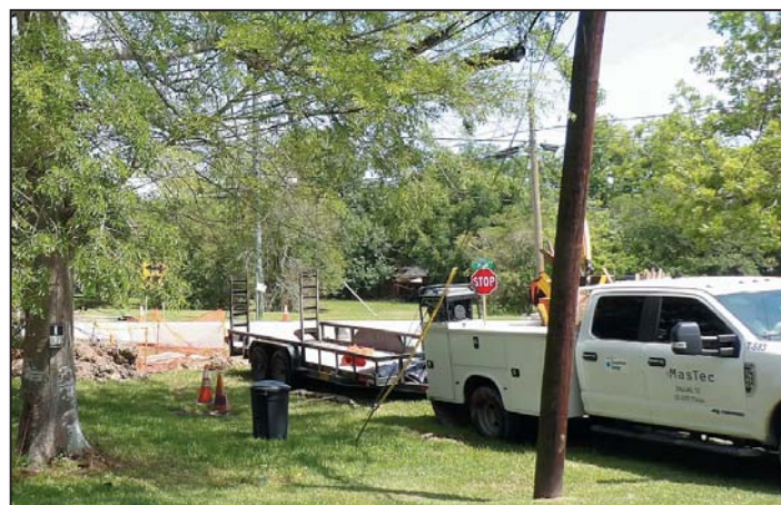
Center Point Energy has begun the digging process to put many a leaning and outworn above ground power line underground where it is immune to wind and jacketed in insulating yellow tube resistant to water saturation for Crosby neighborhoods including old Crosby above.
