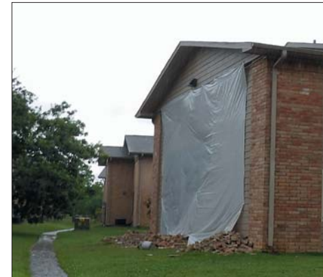
Damage to the apartments included the bricks on building B and in one account a woman was tossed a few feet, although it was not caught on camera. The storm rapidly went north again but no reports of damage were filed in that direction although some small homes lie in that direction. Meteorologists stated that there was no indication of the tornado that was caught on surveillance cameras. But then, it had been reported that there were no tornadoes generated during Hurricane Ike although numerous reliable accounts reported seeing a massive one in Highlands and trees in the reported location were twisted and a Little League Baseball building had its roof twisted off.
