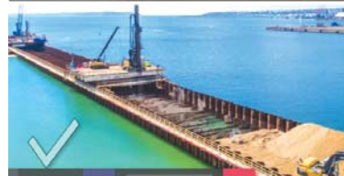
SINGLE WALL COFFERDAM, TOP, WON'T WORK. DOUBLE WALL BELOW IS NEW DESIGN.
