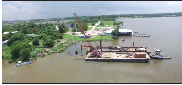
Several work barges, with cranes and other excavation equipment, are anchored along the bank near the San Jacinto River Estates neighborhood. They are removing sunken barges and other debris that impede the flow of the river and pose a hazard during flood conditions. Beyond the work barges can be seen the Riverside Inn, to the far left Meadowbrook Park, and to the far right the area for a proposed barge mooring facility. Work on that project has halted due to a question about whether it was properly permitted by the Corps of Engineers. (All photos courtesy of Greg Moss)
