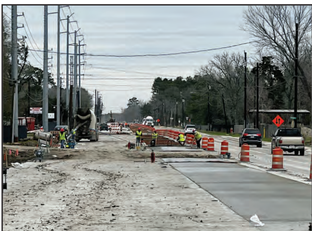
Several contractors are working to widen Crosby-Lynchburg Road from Highlands to Huffman. The 2 lane road will soon be 5 lanes wide.
