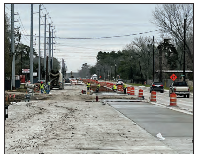
Construction work on the segment between Highlands and Crosby continues, and is scheduled for completion by the 4th quarter of 2023. Like the FM2100 segment, it will be a 5 lane highway, with a median.
