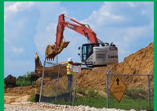
THEA releases a video of current progress at the Southern Impoundment of the SJR Waste Pits.
