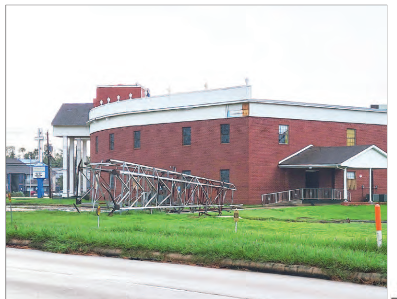
Spirit Of Life Ministries Interdenominational Church on Maxey Road and Woodforest in North Shore lost its steeple, windows were blown out, and the panels from the steeple were blown away from the ferocious winds of Beryl.
