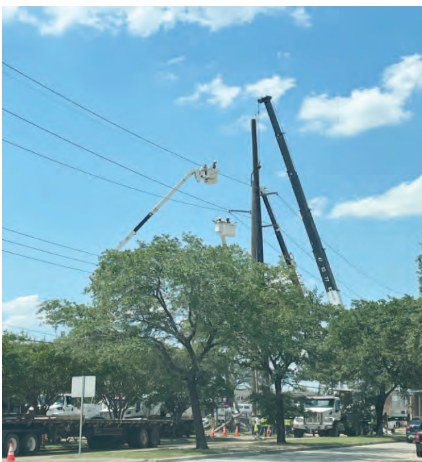
CenterPoint linemen, high in the sky, replace a power pole. This operation took 12 trucks, special drills and crane, and about 20 linemen.
