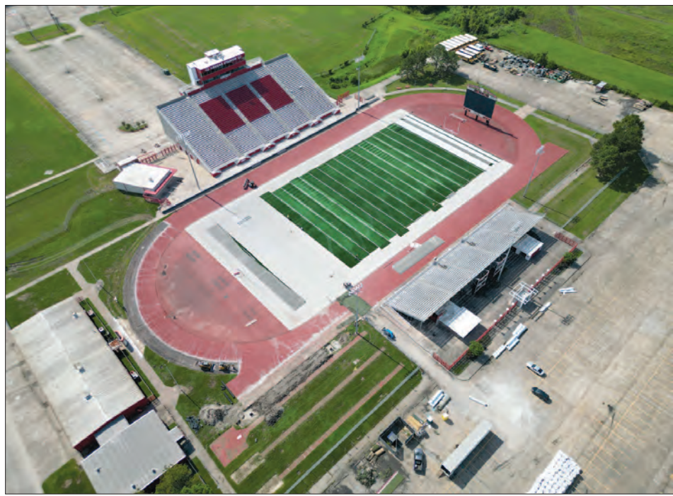
Aerial view of Cougar Stadium. The new turf is being installed and will be ready for the start of Crosby High School's football stadium. Work on replacing the track has also been started. It will be completed following the conclusion of the football season.
