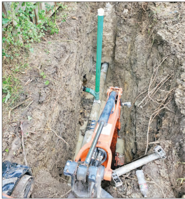
Contractors work on a brand new 8-inch sanitary sewer line located in a backyard easement of a home in Newport Section 6. The sanitary sewer line is at about 9-feet deep and the original line had structural damage that impeded sewage flow so it was pipe bursted from manhole to manhole. This picture shows the contractor reinstalling the homeowner’s connection of sanitary sewer service to the new main line and installing a clean out that indicates where the service connects to the main line. (By David Taylor)
