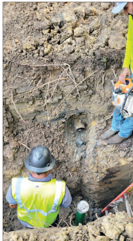
Workers are clamping together the new sanitary line to fully ensure sewage flow will go downstream into the manhole. The clamp is the metal container with blue screws on it. Newport MUD district board members are expected to approve a referendum seeking a bond authorization for $109 million at their meeting this week. (Photo by David Taylor)
