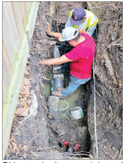
This homeowner's sanitary sewer service is exposed and the workers are reconnecting it to the new sanitary sewer line. Work on the lines throughout the district are constant. (Photo by David Taylor)
