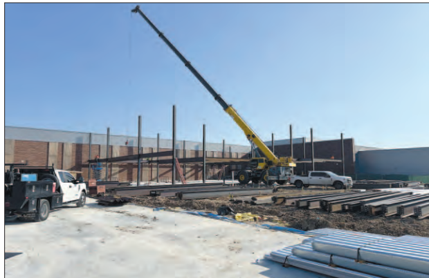
The foundation has been poured and now steel columns are going up for the new academic wing at Crosby High School. The expansion will 32 classrooms and 8 labs to CHS. The project is expected to be completed in late fall of 2025.
