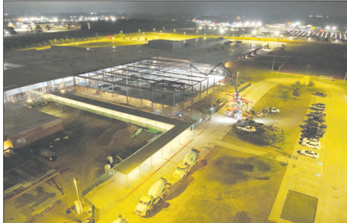
On November 1, crews completed the final concrete pour for the second floor of the new academic wing at Crosby High School. The CHS expansion project, including the new academic wing and expanded welding and carpentry labs, will increase classroom space inside the high school by 50%. The project is expected to be completed in the fall of 2025. It is funded by bond monies approved by voters in 2017.
