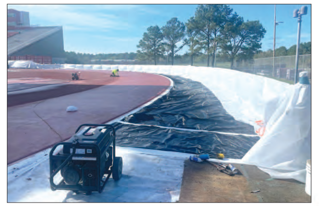
Construction crews are finalizing the track resurfacing at Cougar Stadium. This is the final phase of the turf and track replacement at the stadium.
