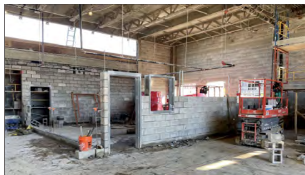
Photo of carpentry lab currently under construction in the Crosby High School expansion.
