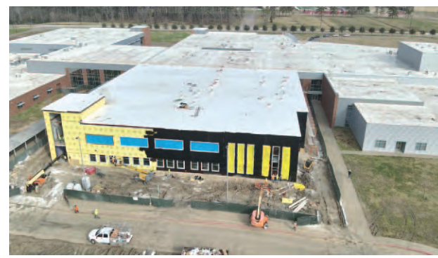
Drone photo above new academic wing being built at Crosby High School. The new academic wing will contain 32 classrooms and 8 labs, increasing the learning space inside CHS by 50%.
