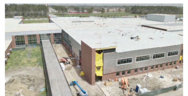
Exterior of the new academic wing at Crosby High School. Weather-proof panels have been installed on the exterior of the addition, and now construction crews are applying brick to match the current façade of CHS. Crews are 95% finished with the installation of doors and windows.
