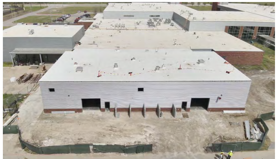
Exterior of the expanded CTE (Career and Technical Education Center) at Crosby High School. This building will house additional welding and carpentry labs. In all, the CHS expansion is increasing classroom and lab space by 50% inside CHS.
