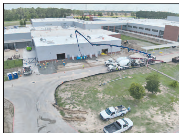
On June 17, construction crews poured the final concrete for the lip of the expanded CTE (Career and Technical Education) Center as part of the new Crosby High School expansion. The CTE expansion is on the foreground. The new academic wing is just behind the bus portico. The new academic wing will feature 32 classrooms and 8 labs with room for an additional 912 students, bringing the functional capacity of CHS to 2837 students.
