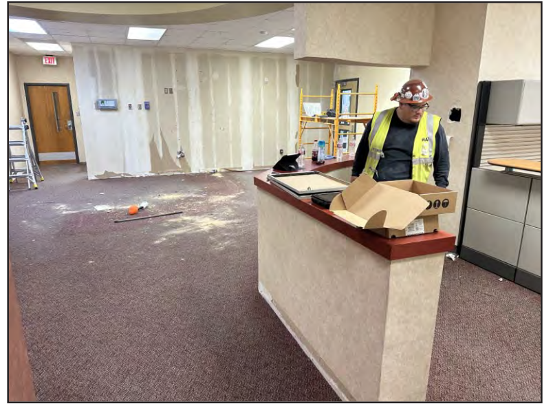
Construction projects are happening at each campus in Crosby ISD during the summer break. Inside Drew Elementary School, the entire front office area is being redesigned with several safety upgrades.
