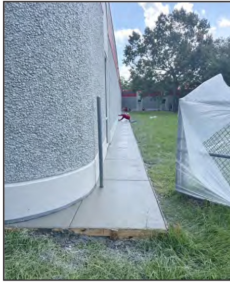
Construction crews are adding playground upgrades at each elementary campus in Crosby ISD. At Newport Elementary School, crews have added a new concrete lip around the perimeter of the school.
