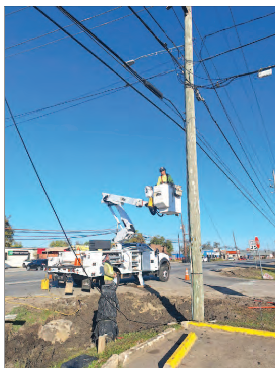
CenterPoint crews were up and down FM 2100 all last week working on adding 58 new streetlights.
