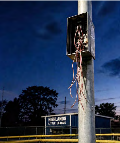
Copper wiring hangs from a damaged electrical box at Highlands Little League after thieves reportedly broke into the ballpark and stole electrical connections. (Photo from Highlands Little League facebook page)
